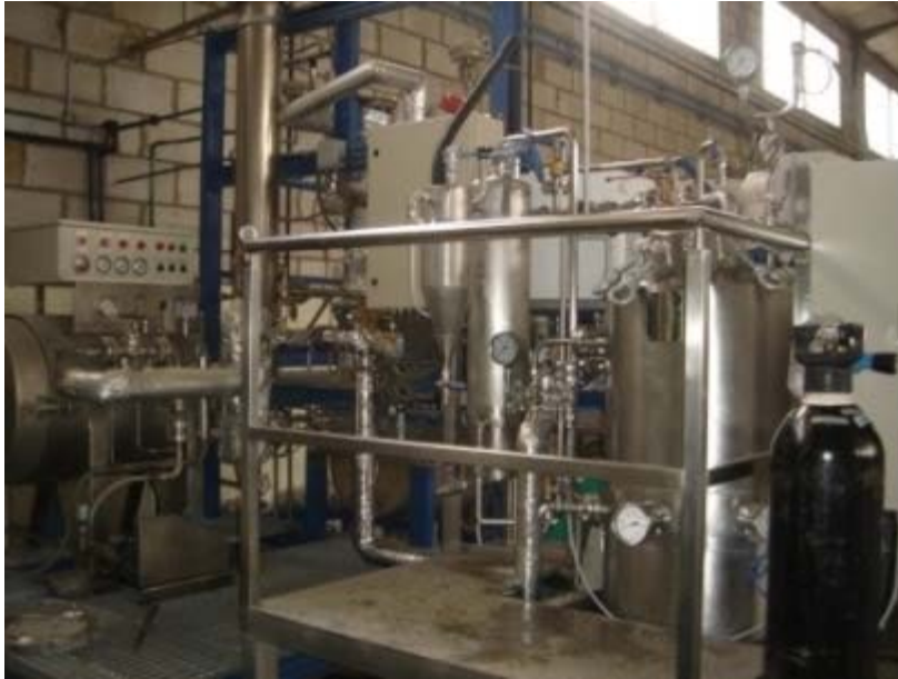
Figure 8: Semi-pilot steam explosion system (IG Pilot plant)
