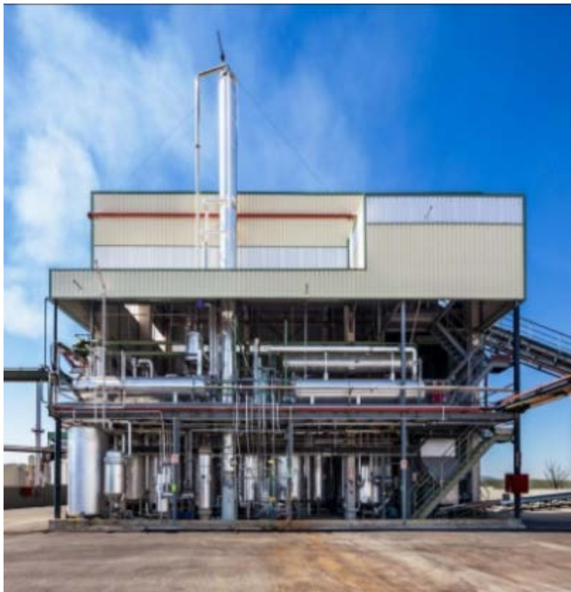
Figure 2: Oleicola El Tejar – NATAC extraction plant
