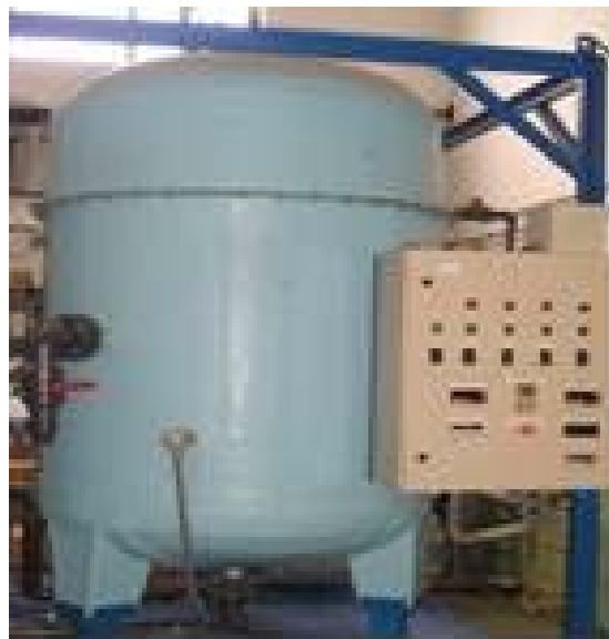
Figure 6: Anaerobic reactor (IG Pilot plant).
