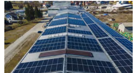
Solar power plant with a capacity of 437 kW at the ESOF business facility installed in 2021 (Source: radiodonjivakuf)
